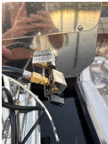
Grill valve and regulator detail
