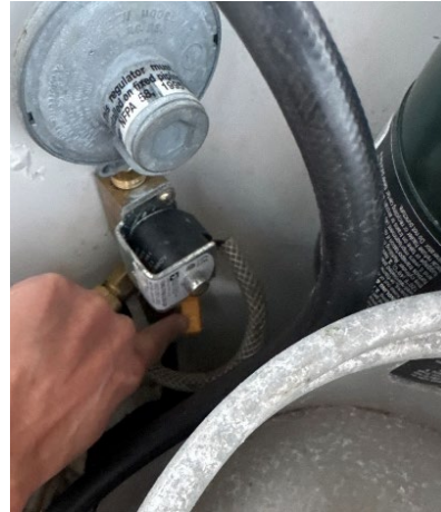
Propane valve inside the locker — push down on the yellow valve to open
